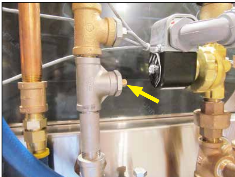
Fig. 21 - Rinse-aid injection point.
