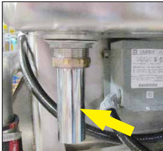
Fig. 7 - 1-1/2" scrap sink drain.
