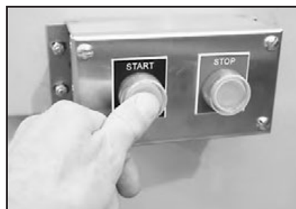
Start/Stop Station ON.
