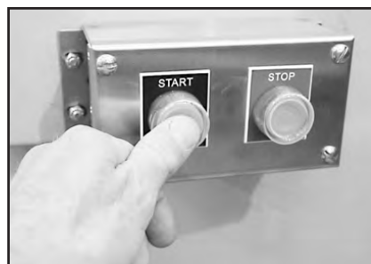
Start/Stop Station ON.
