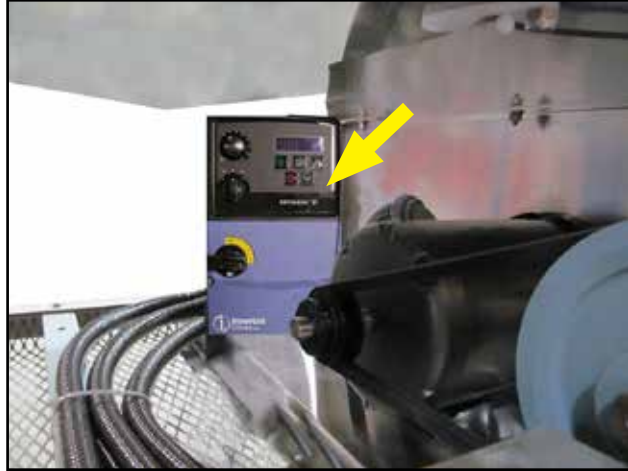
Fig. 7 - The VFD is located behind the drive motor.
