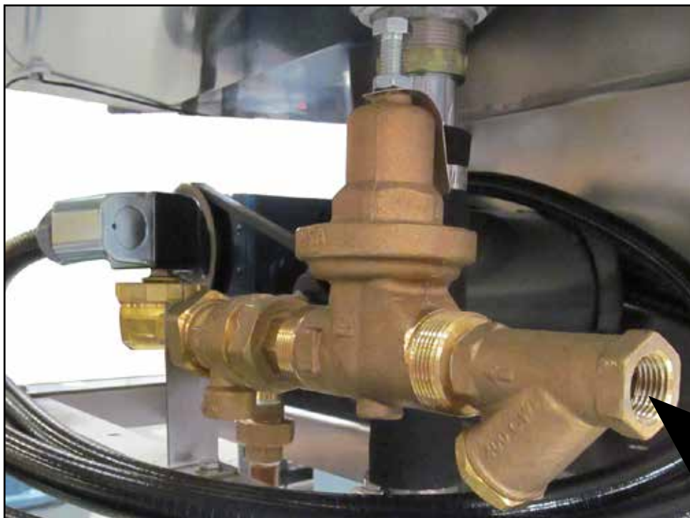
Fig. 21 - DWT 1/2" NPT cold water connection.
